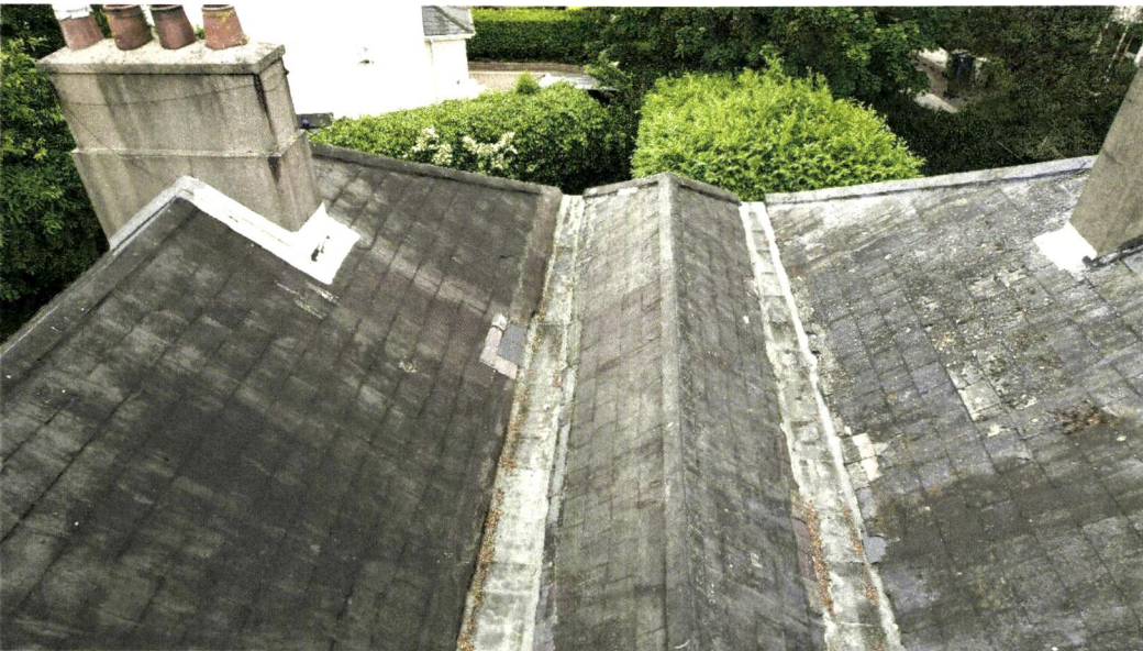
Two long valleys – note the repairs in the valley and around the chimney stack
