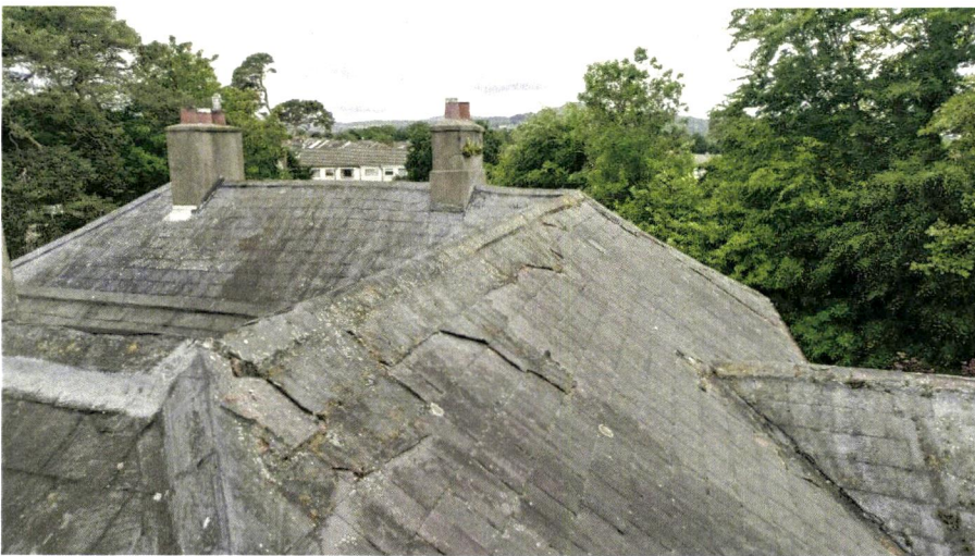
Poor condition of the main roof and the use of bitumen over the slates
