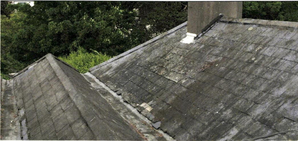
Slates that have been repaired on the roof. In addition many of the slates have slipped and are broken
