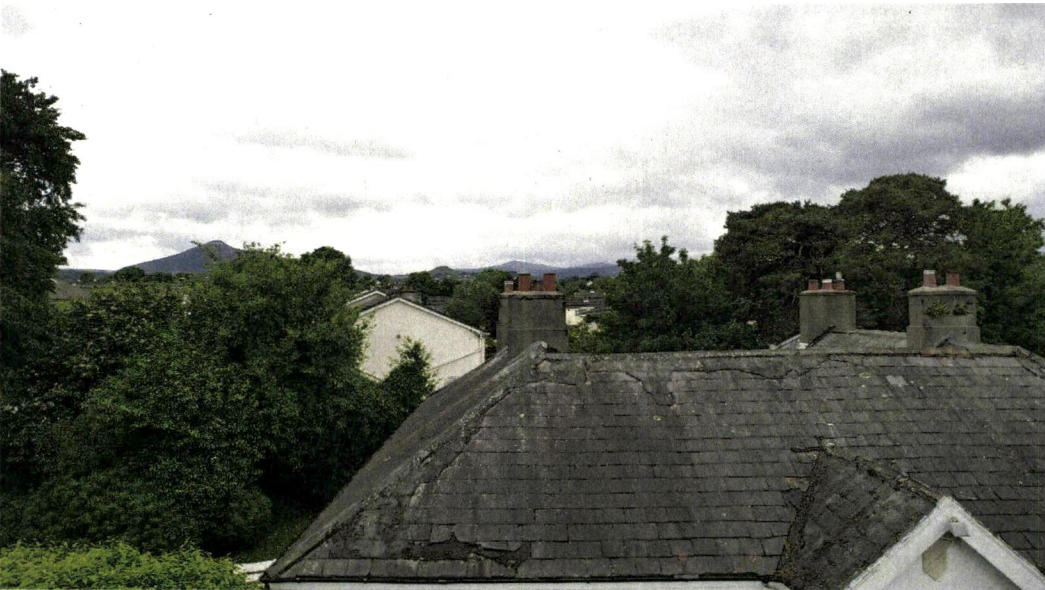
Repairs around the hip at the front of the roof and over the ridge with bitumen. These slates are not salvageable
