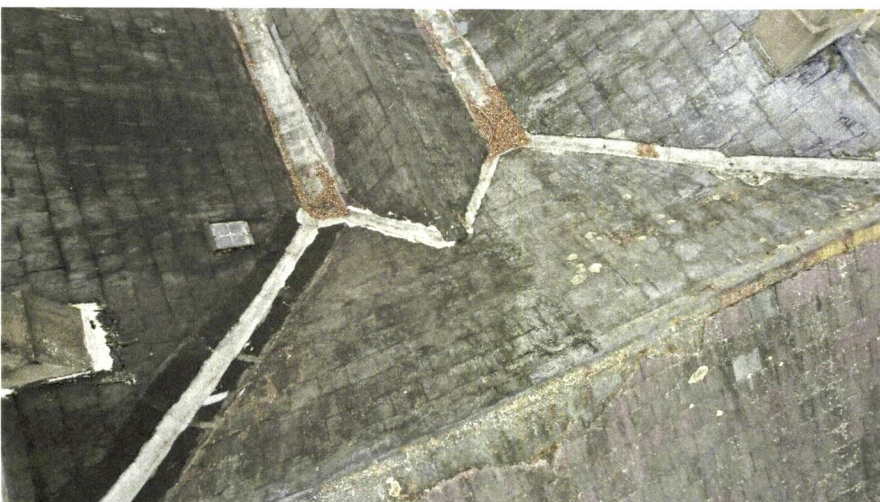
Roof valleys – note the valley on the left which has bitumen on the valley- also note the skylight access to the roof
